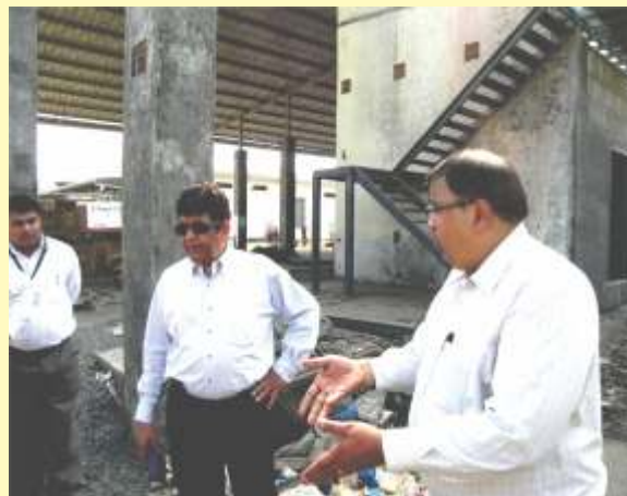
Shri Hasmukhbhai seen in a serious discussion with Shri Mahendra bhai during construction in progress at the Vapi Super Hub
